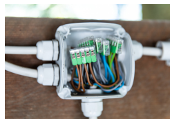
Wiring in the distribution box
